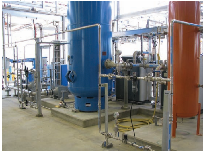
Western Corridor Recycled Water Project, SE Queensland
